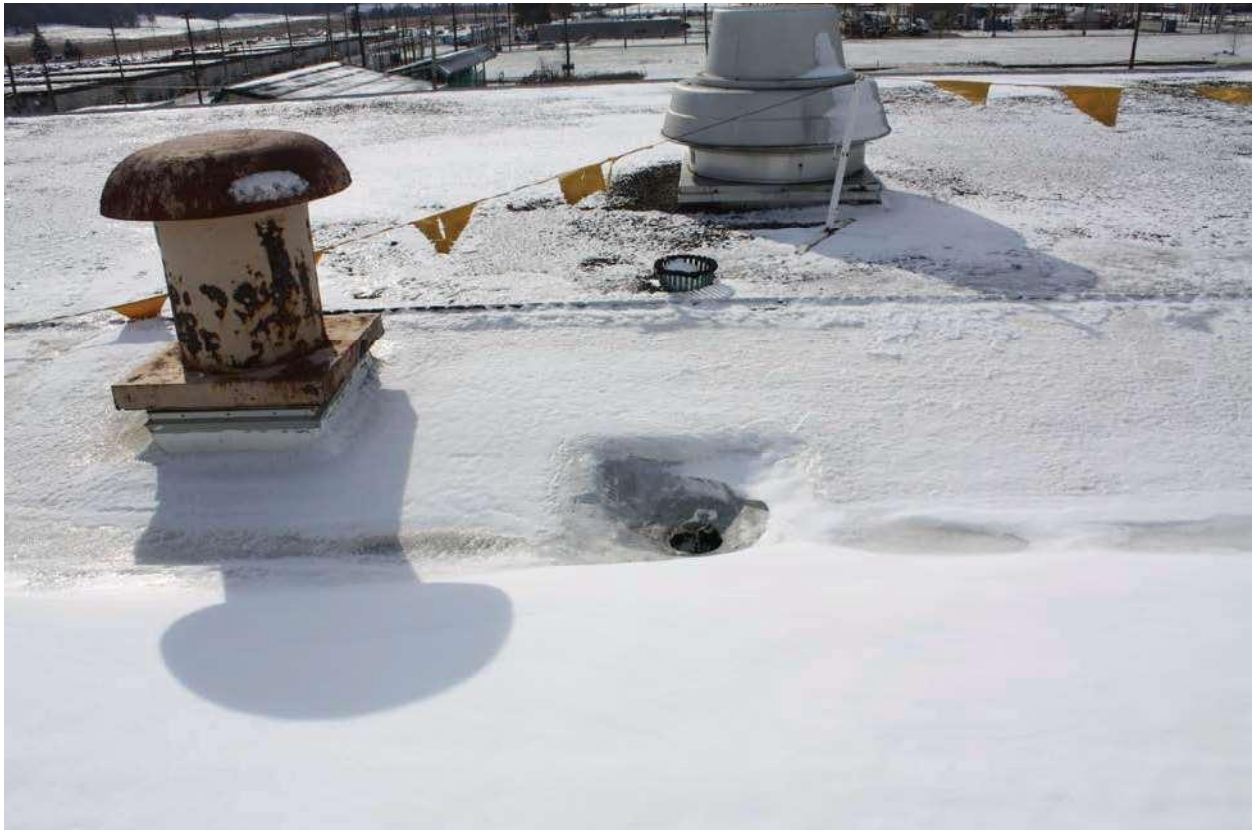
Looking South – Roof Drain Screen to be Replaced on Highbay Roof
