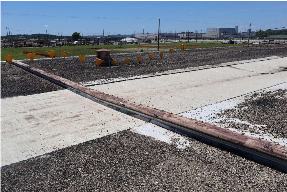
Main Low roof– Bare spot by expansion joint
