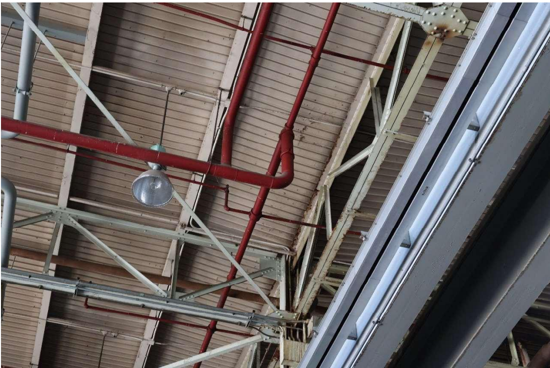
Minor corrosion on beam near K9
