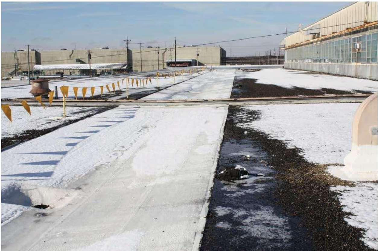
Looking West – Drain Screen Needs Replaced
