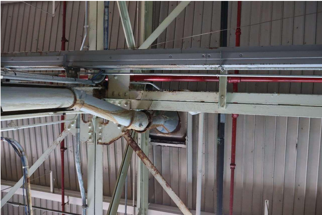
Roof at column B15 where the leak is coming from
