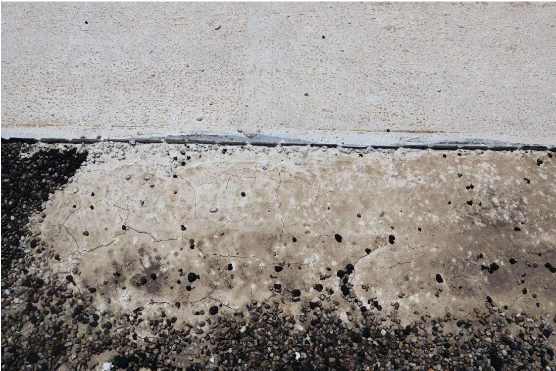
Main Low roof – Small cracks in Overlay
