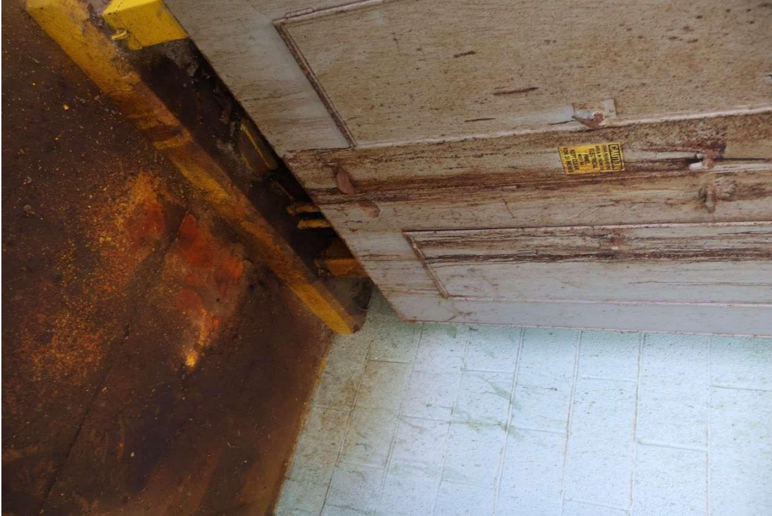
Evidence of leak at column K17
