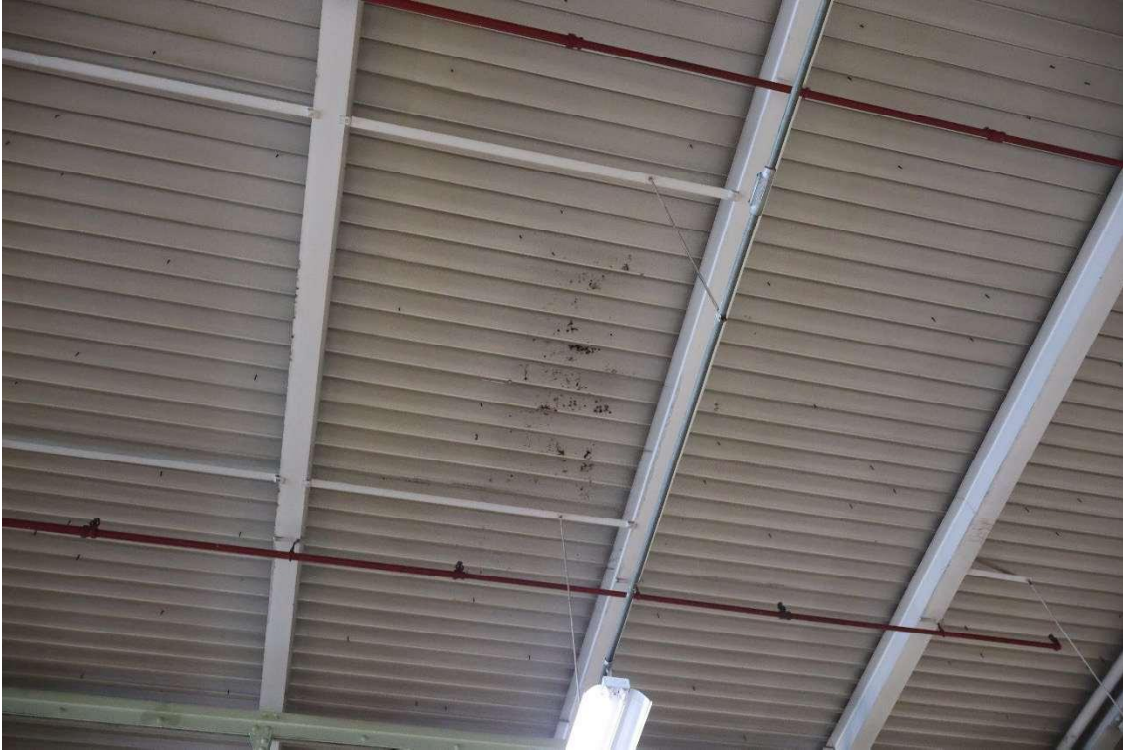
Minor surface corrosion in Respirator Facility
