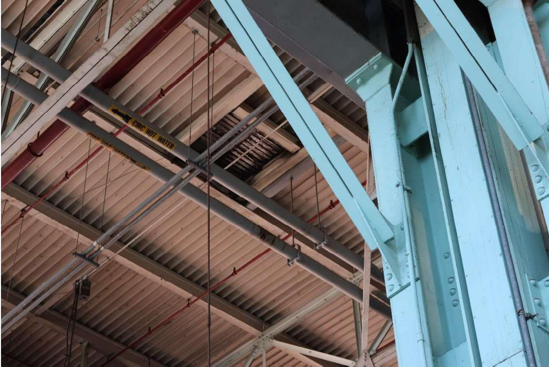
Leak stains on pipes near column K2
