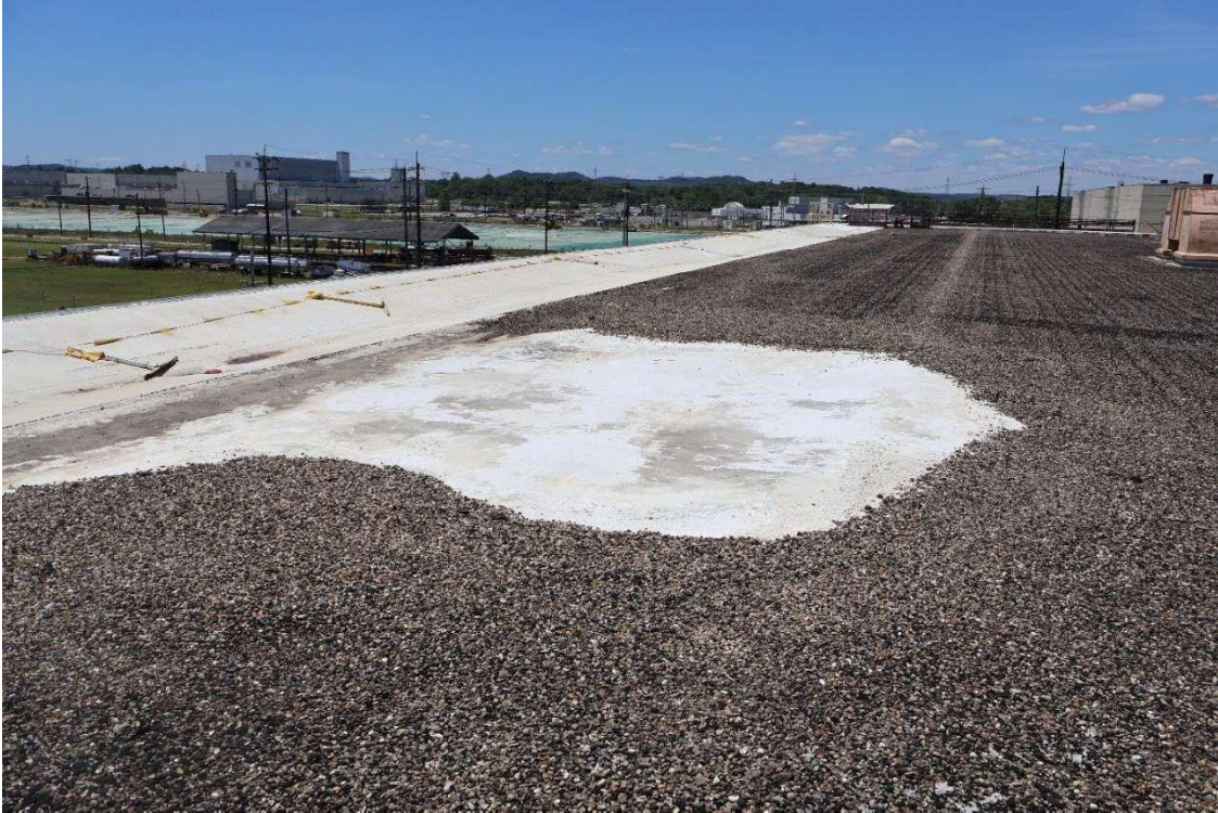
Main High roof – Large bare spot
