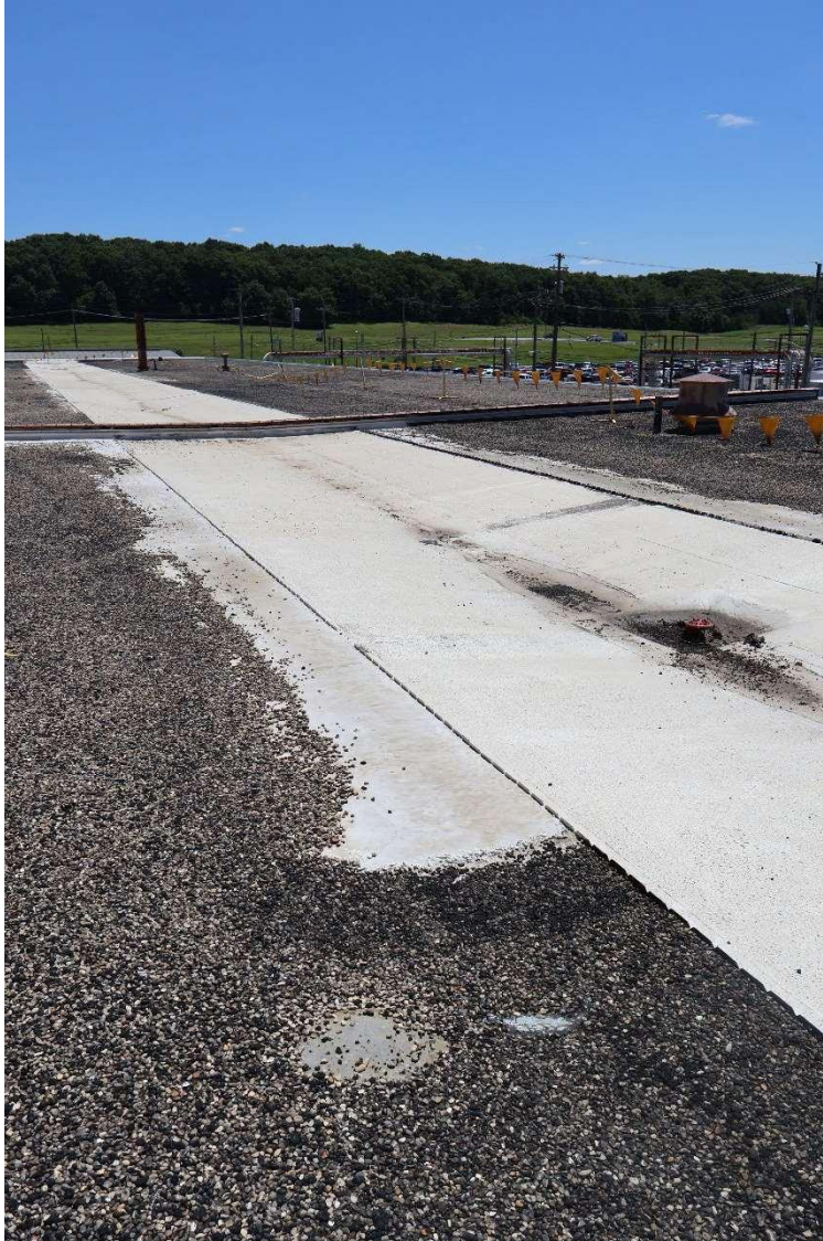
Main Low roof – Valleys shown and bare spots
