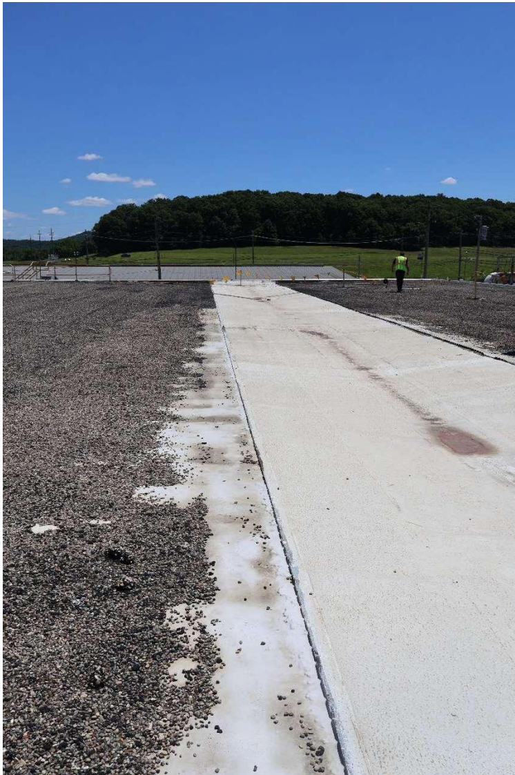
Main Low roof – Valley shown and bare spots
