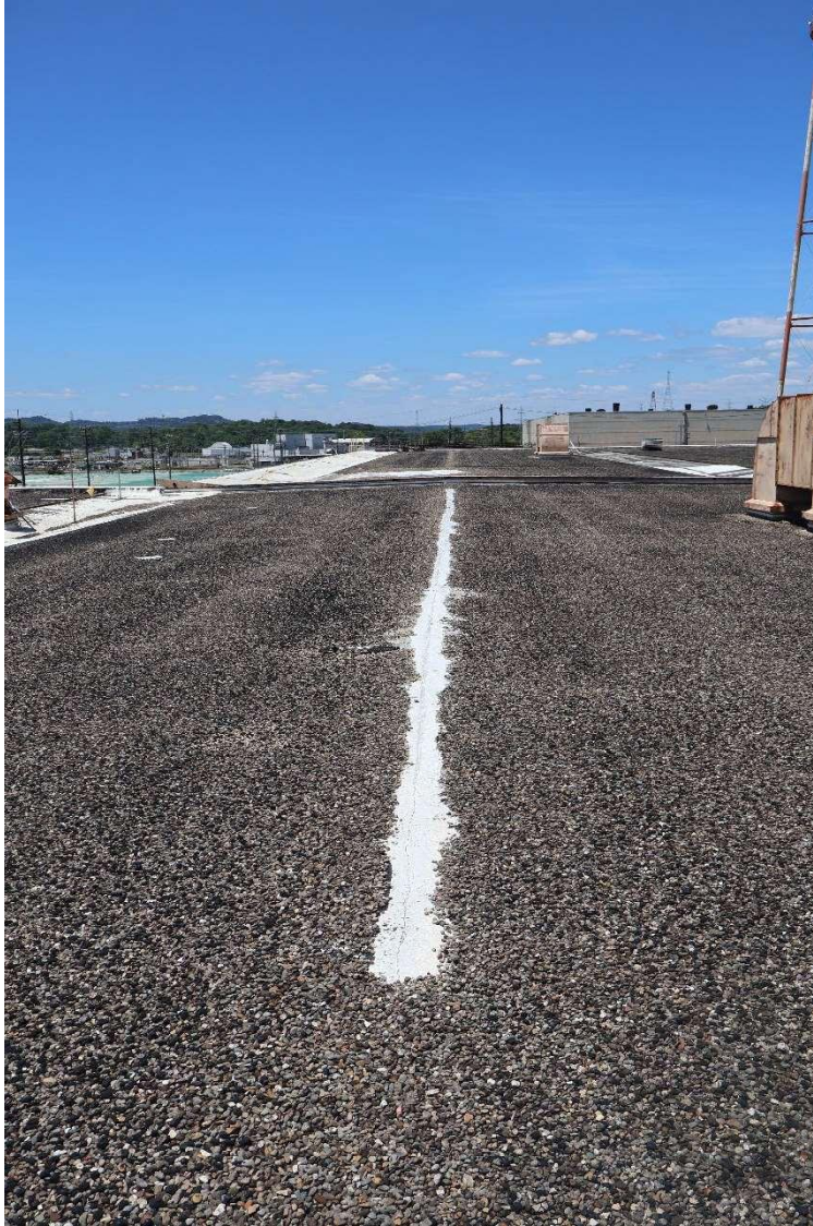
Main High roof – Bare spot in gravel along ridge
