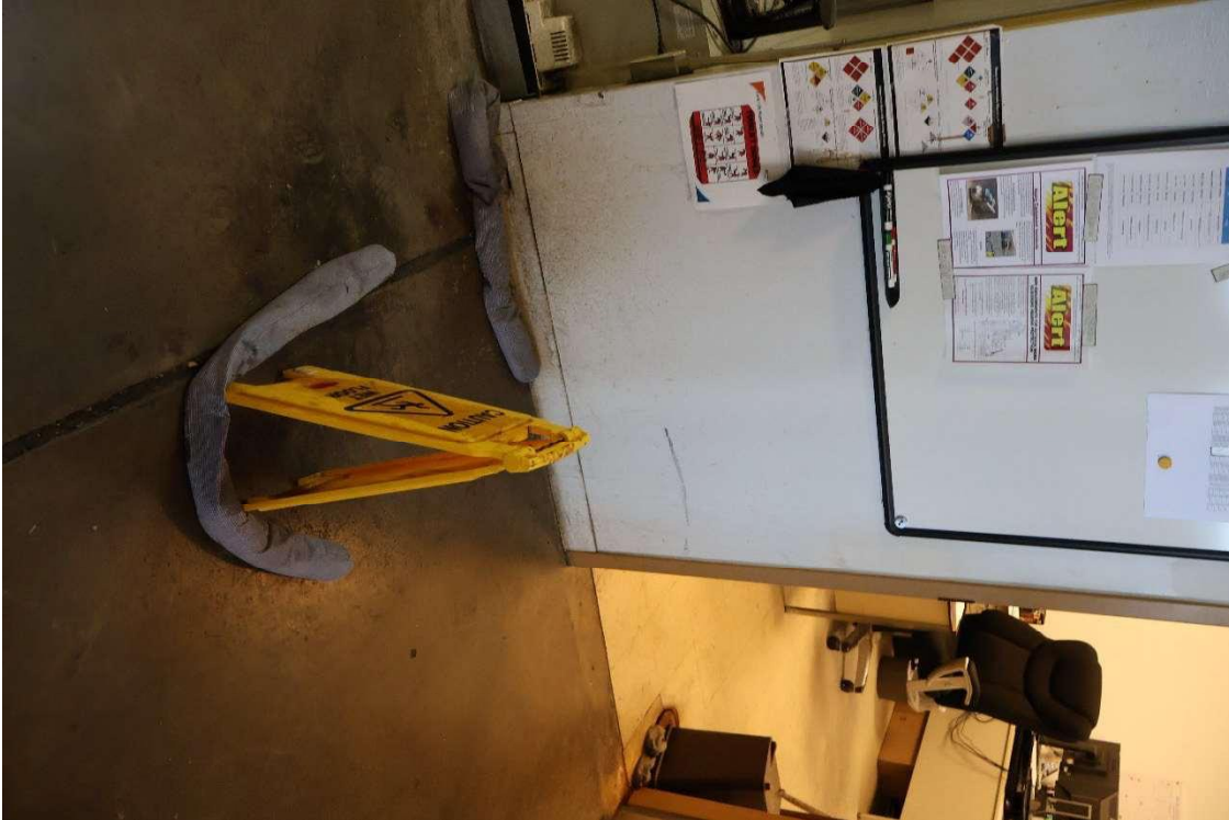
Leak near column C14
