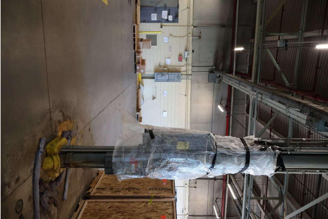
Water damage at column B15
