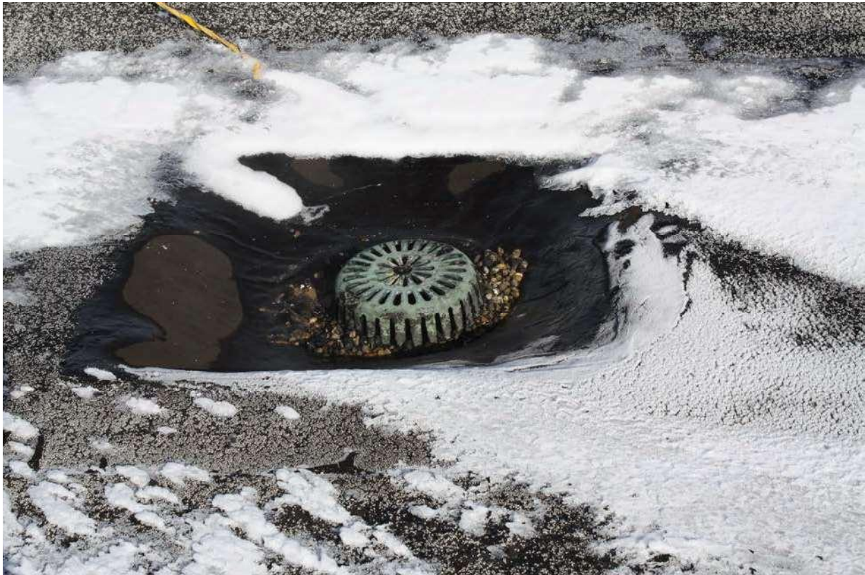
Highbay Roof Drain – Gravel Present at Drain to be Removed, Common
