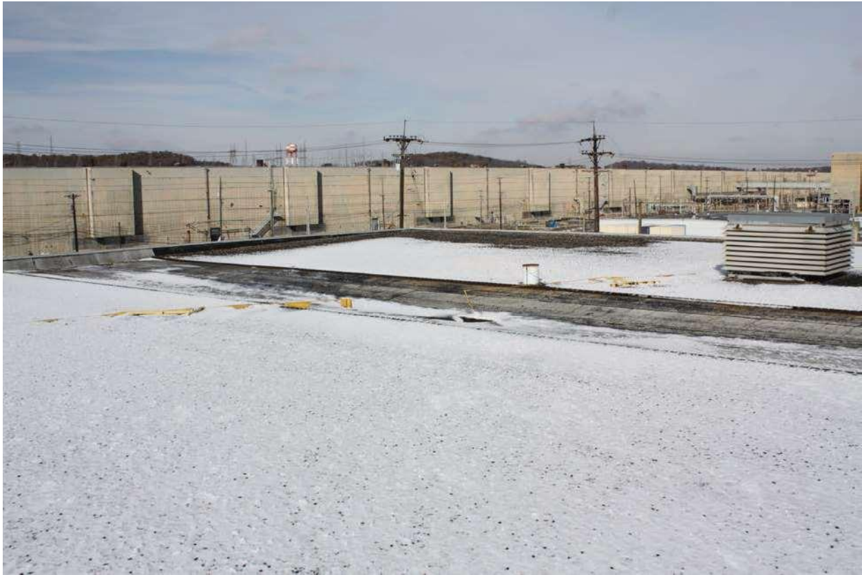
Looking Northwest – Highbay Roof, Stanchions to be Corrected
