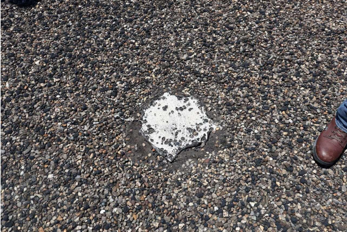
Main High roof – Possible repair/patch work
