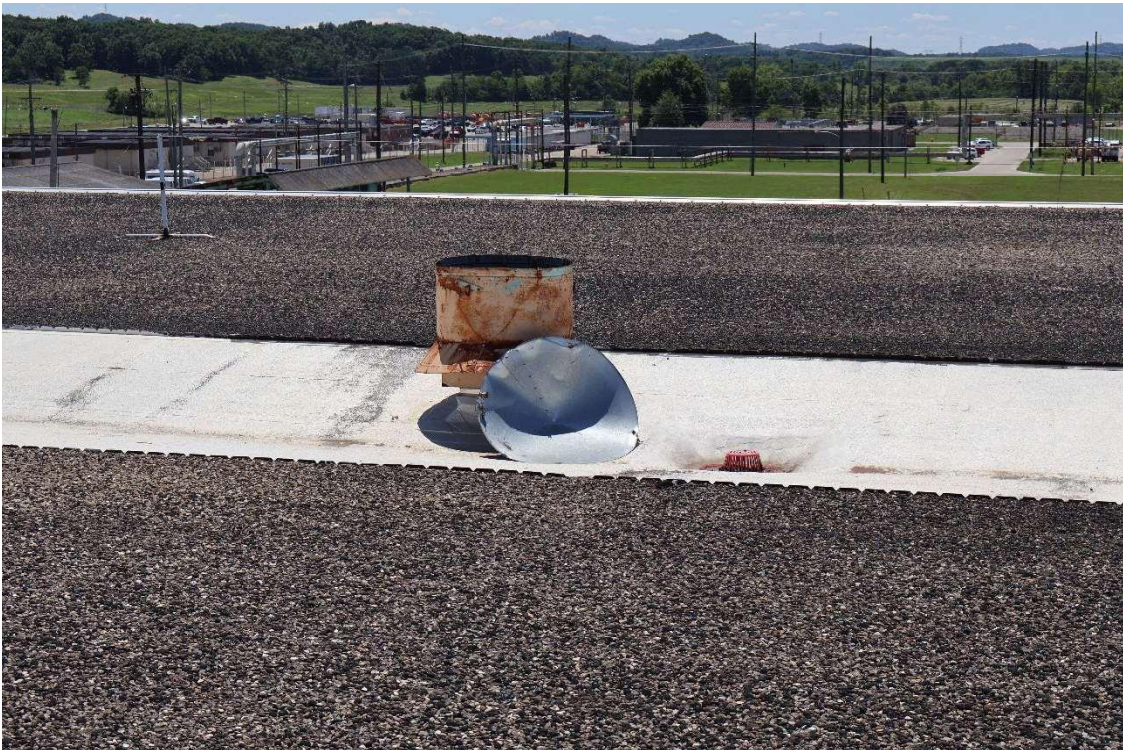
Main High roof – Loose debris broken off from vent
