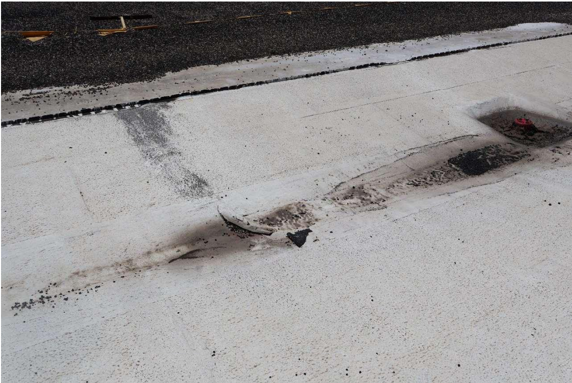
Main Low roof – Damage in the Overlay in the valley
