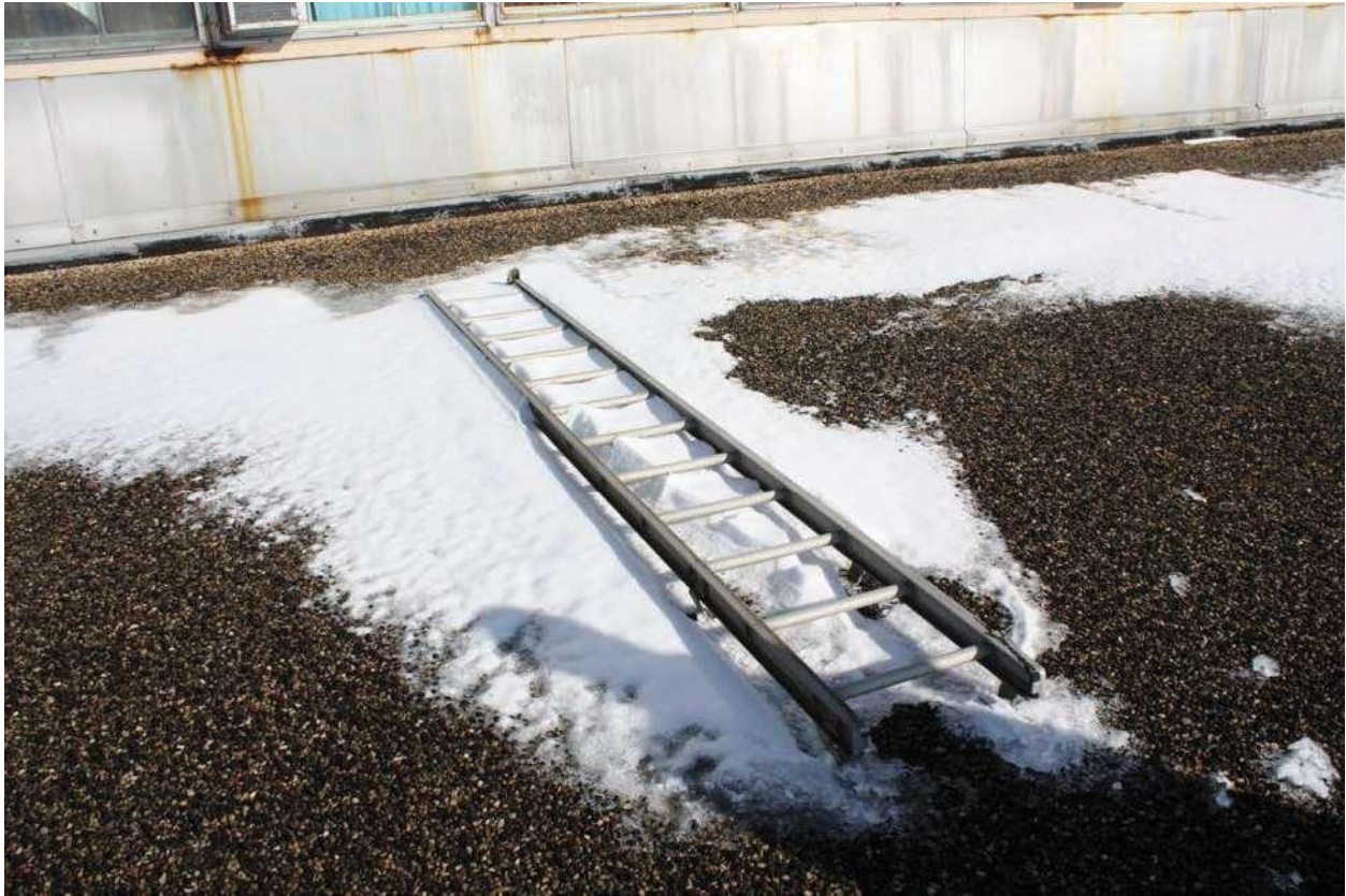
Debris to be Removed from Main Low Roof
