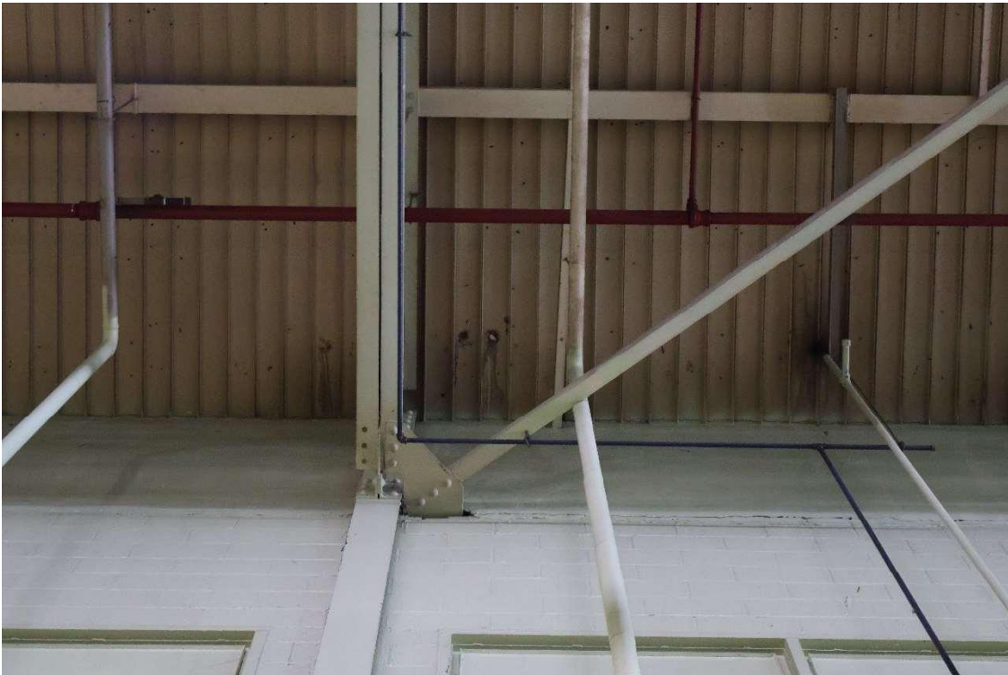
Minor holes near column D7
