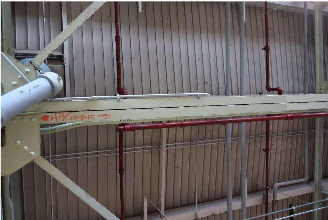
At column B10 where there is a leak
