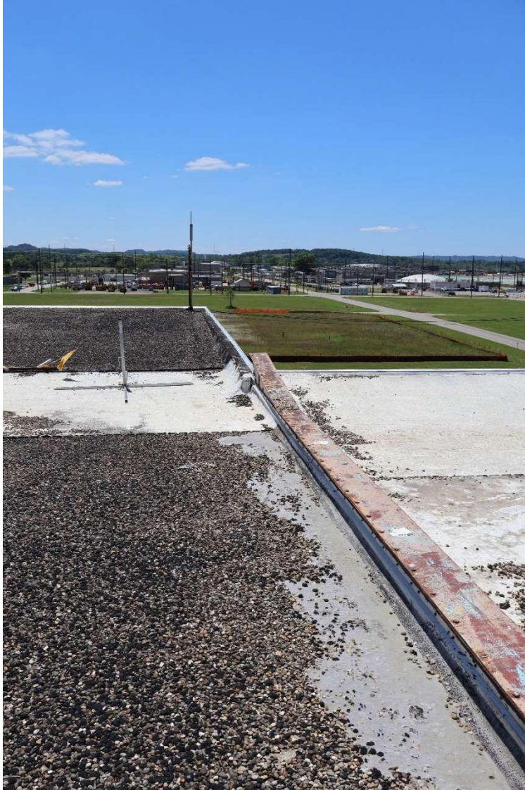
Main High roof – Expansion joint cover on South side is not secured
