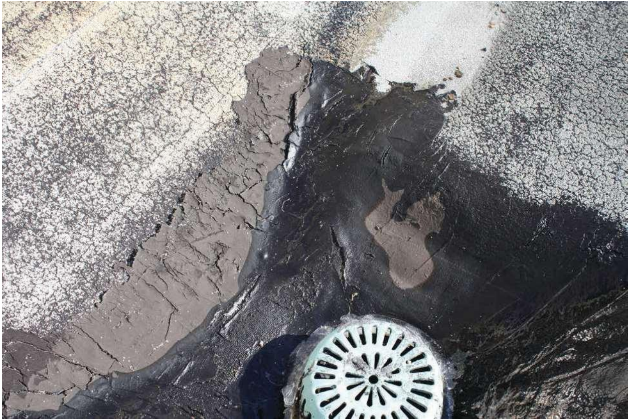
Minor Cracking at Roof Drain – Main Low Roof
