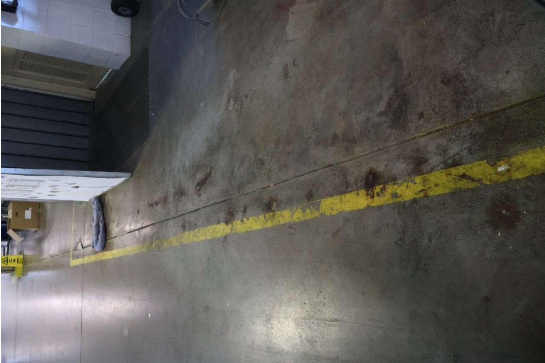
Evidence of leaks near column B13
