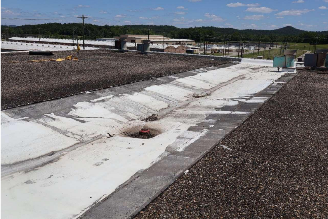
Main High roof – Gravel in the valley from runoff
