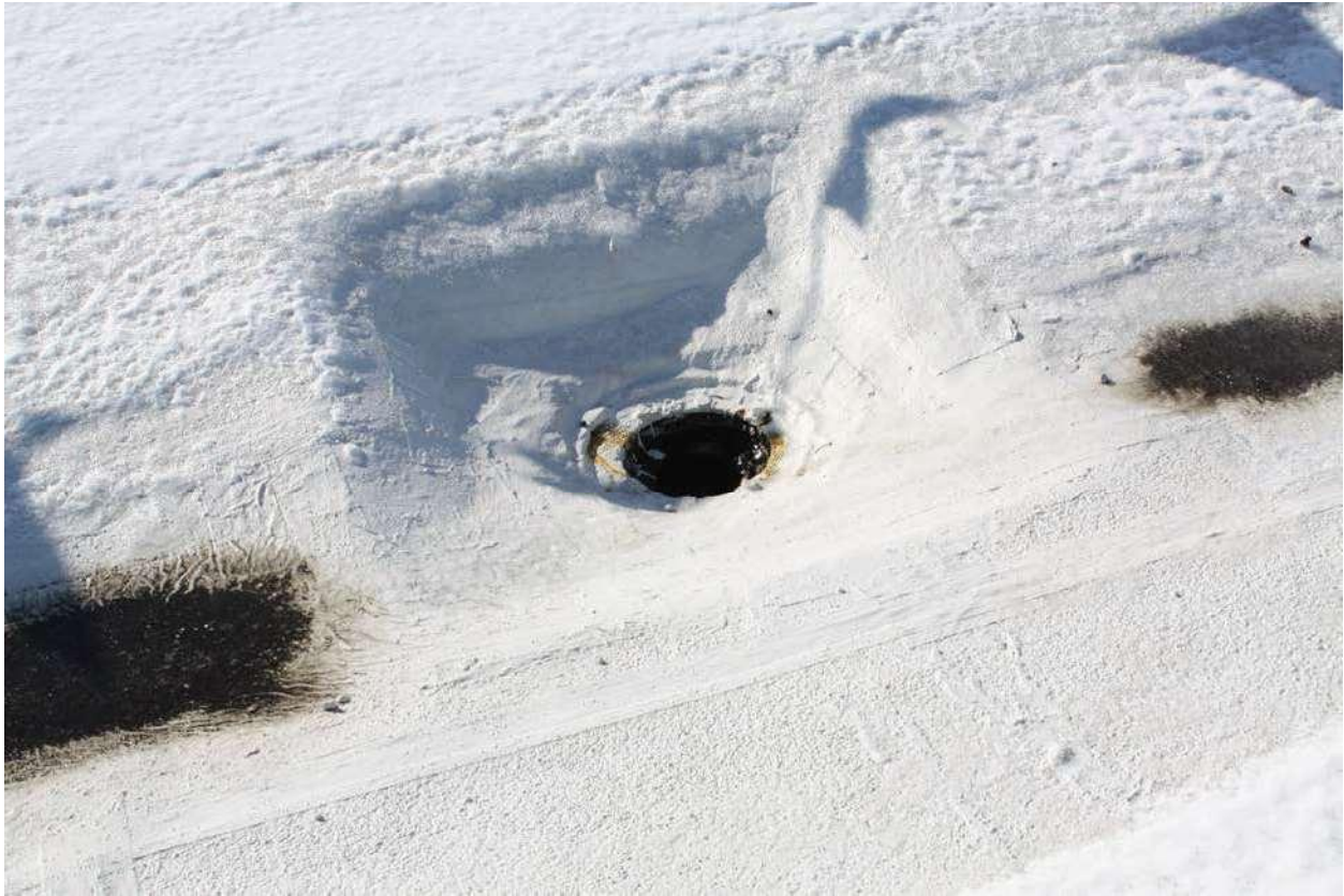
Main Low Roof – Missing Drain Screen
