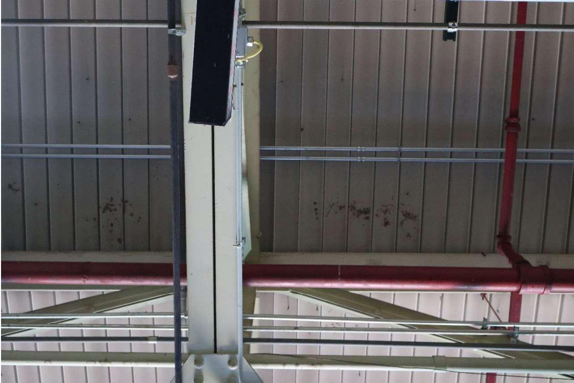
Light surface corrosion near column B14
